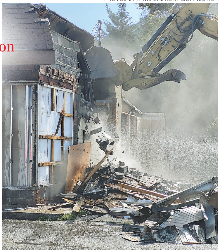
Demolition equipment tears down the walls at 8249 Richmond Highway in Mount Vernon.
